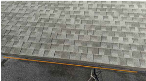
Missing transition Flashing
