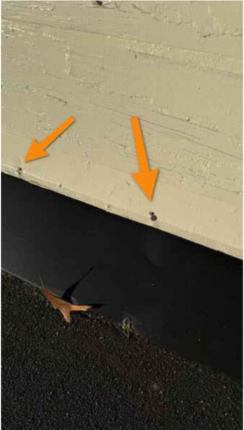
Holes in flashing.
