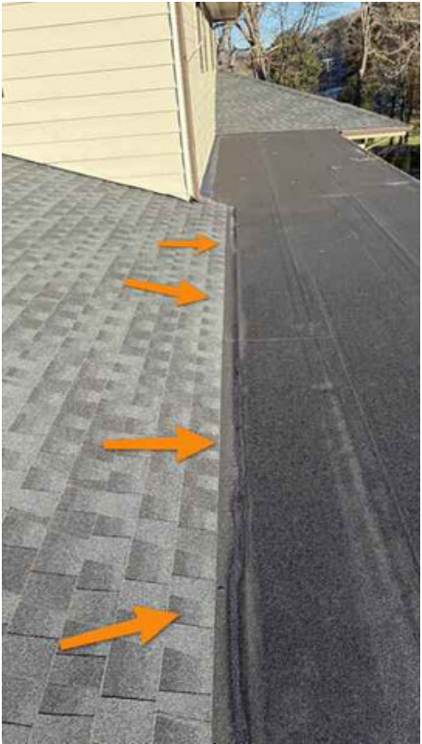
missing transition flashing.
