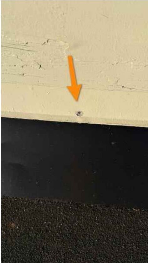
Holes in flashing.
